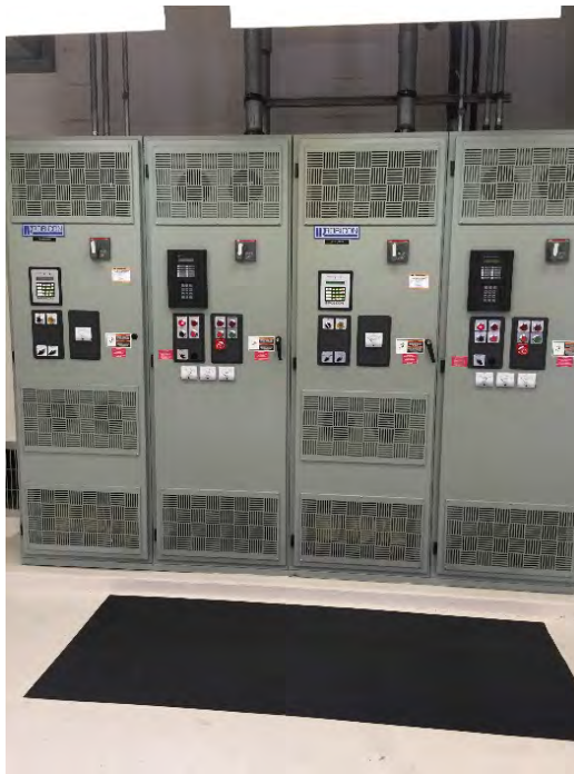
Photo 4.48 - Effluent Pump Station Variable Frequency Drive Nos. 4 and 5
