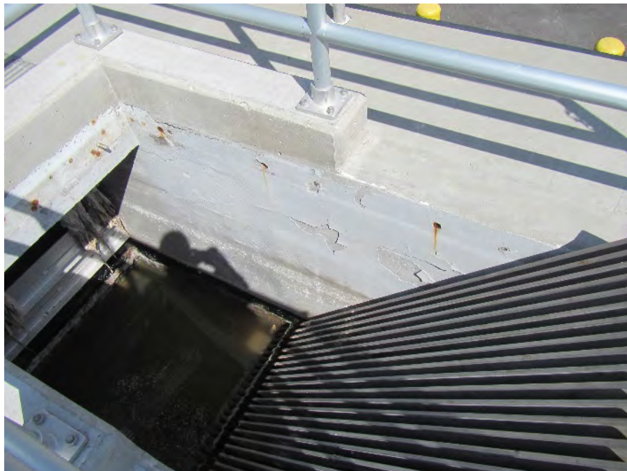
Photo 5 - Coating failure has occurred in the inlet and outlet channel at the manual Bar Screen
