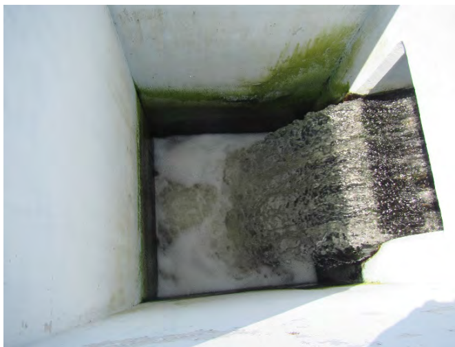
Photo 4.27 - Secondary Clarifier Discharge
