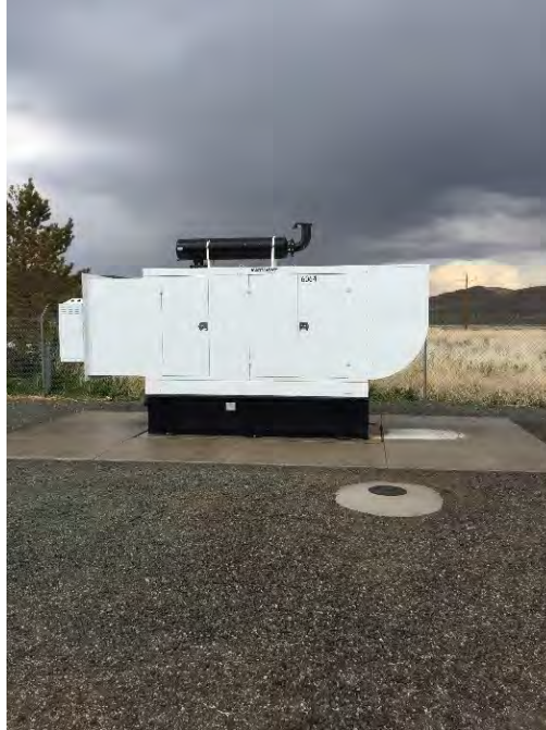
Photo 4.4 - SCLS Backup Emergency Diesel Generator
