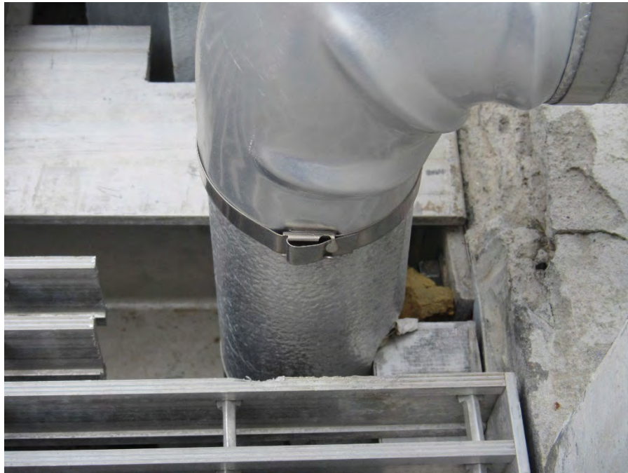
Photo 19 - Minor Concrete cracking at the Chlorine Contact Basin
