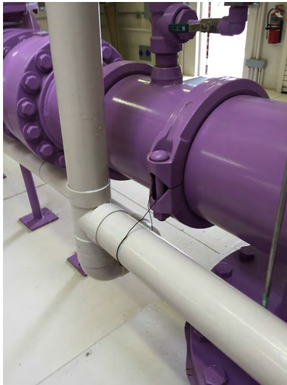
Photo 20 - Pump and piping drains are supported by rope or wire
