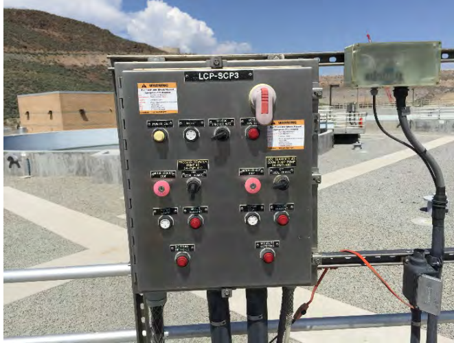
Photo 4.25 - Clarifier No. 3 Local Control Panel
