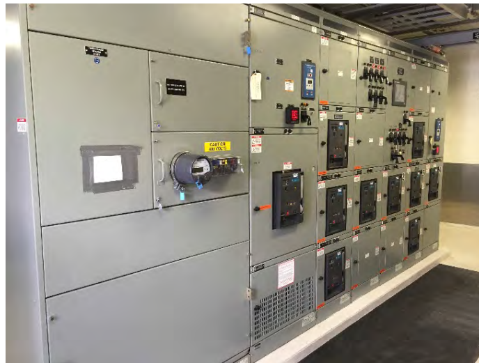
Photo 4.32 - Blower Electrical Room
