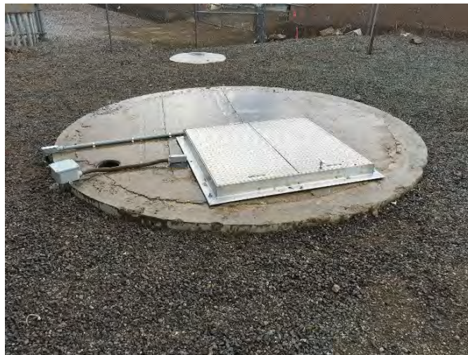
Photo 4.1 - SCLS Wet Well
