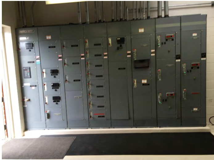
Photo 4.46 - Effluent Pump Station Electrical Room
