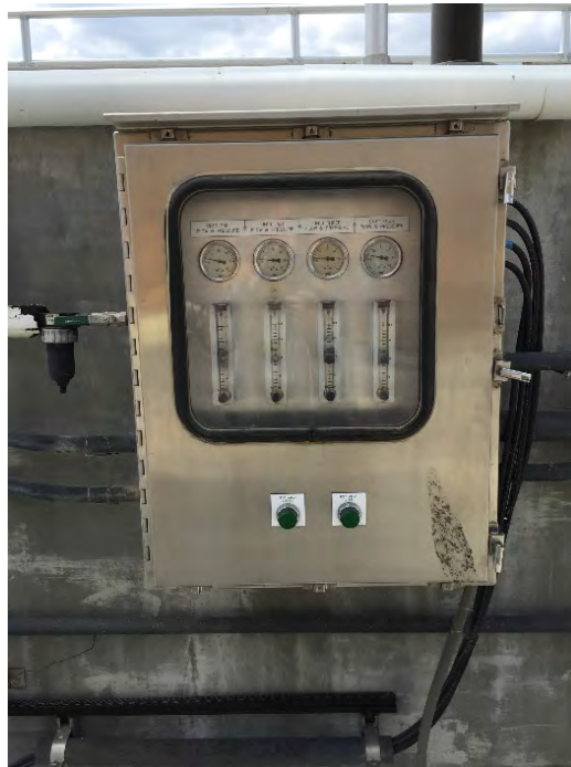
Photo 4.31 - Air Lift Pump Instrumentation
