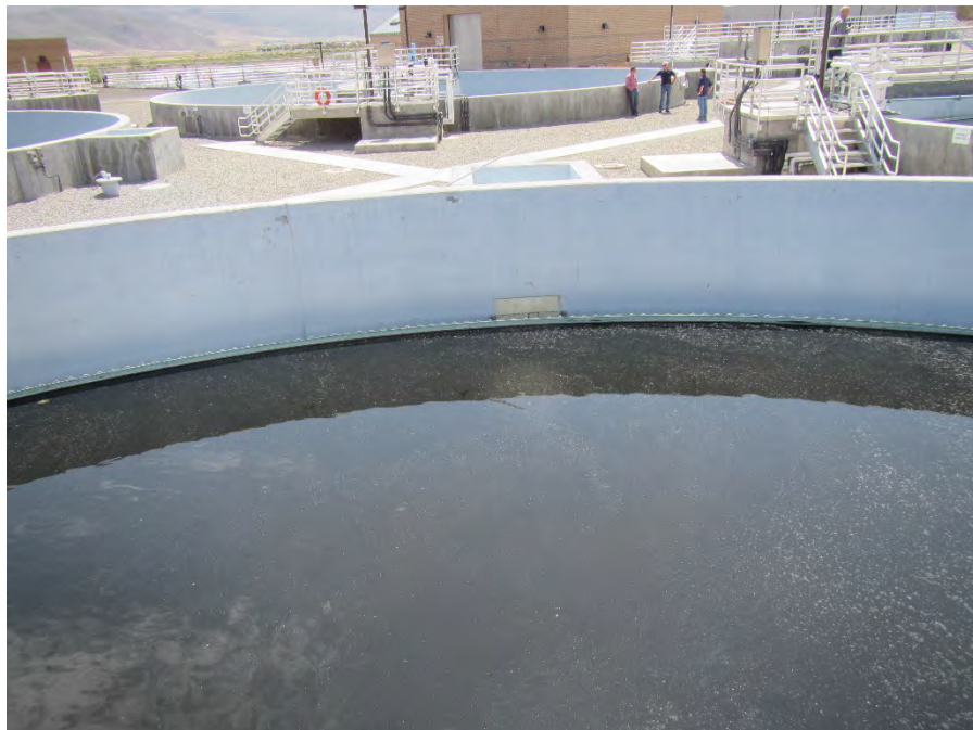
Photo 14 - Coating failure has occurred Secondary Clarifier No 3
