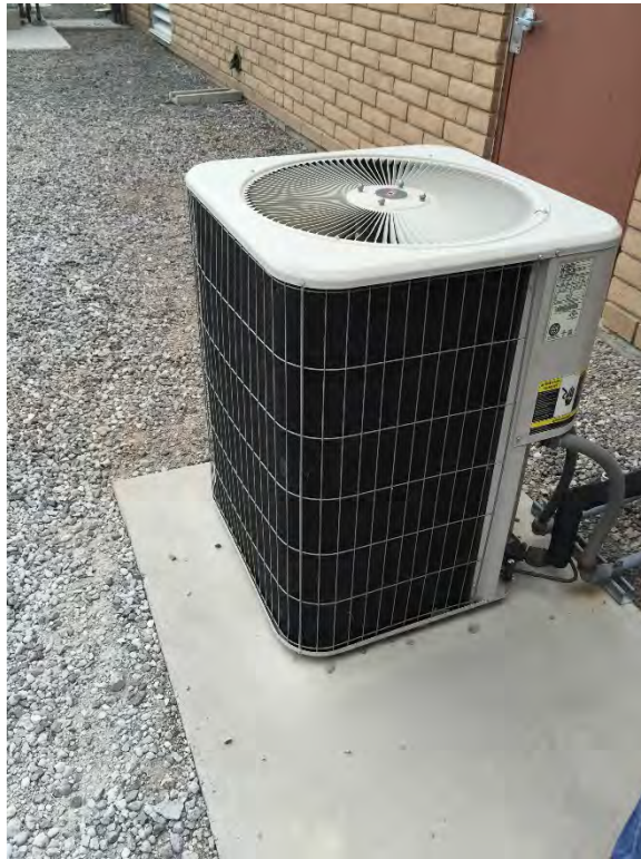
Photo 27 - Effluent Pump Station Electrical Room AC unit often freezes the evaporative coil within the air handler unit-Compressor and Condenser
