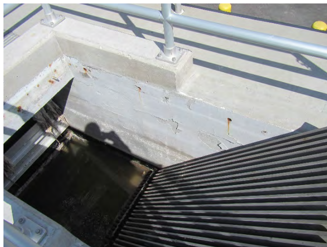
Photo 4.14 - Manual Bar Screen and Channel
