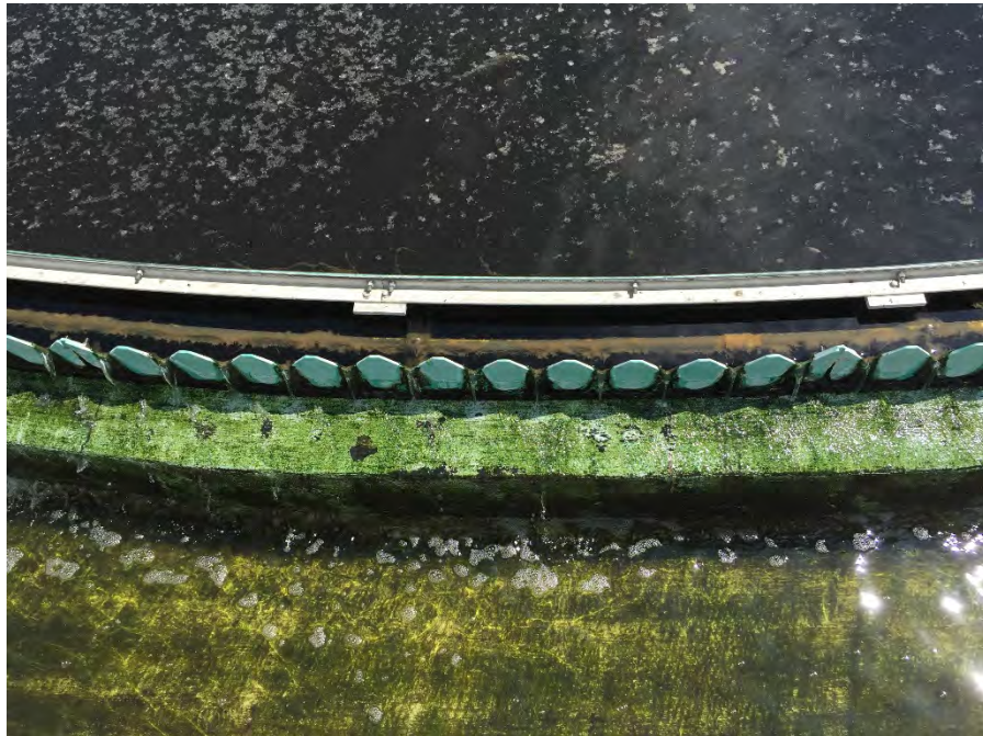
Photo 15 - Algae build up on the launderer V-Notch weirs at the Secondary Clarifier creating a maintenance issue
