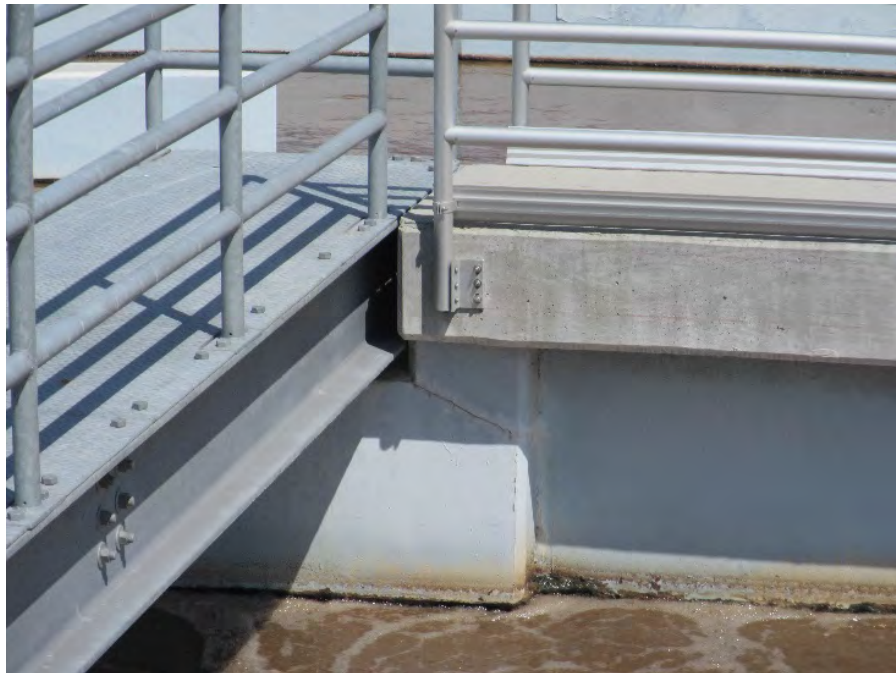
Photo 8 - Cracks at Oxidation Ditch
