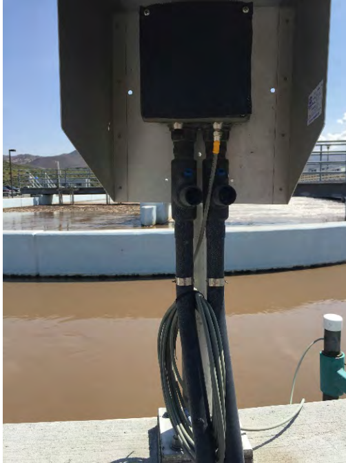
Photo 4.20 - Meter with Sun Shade
