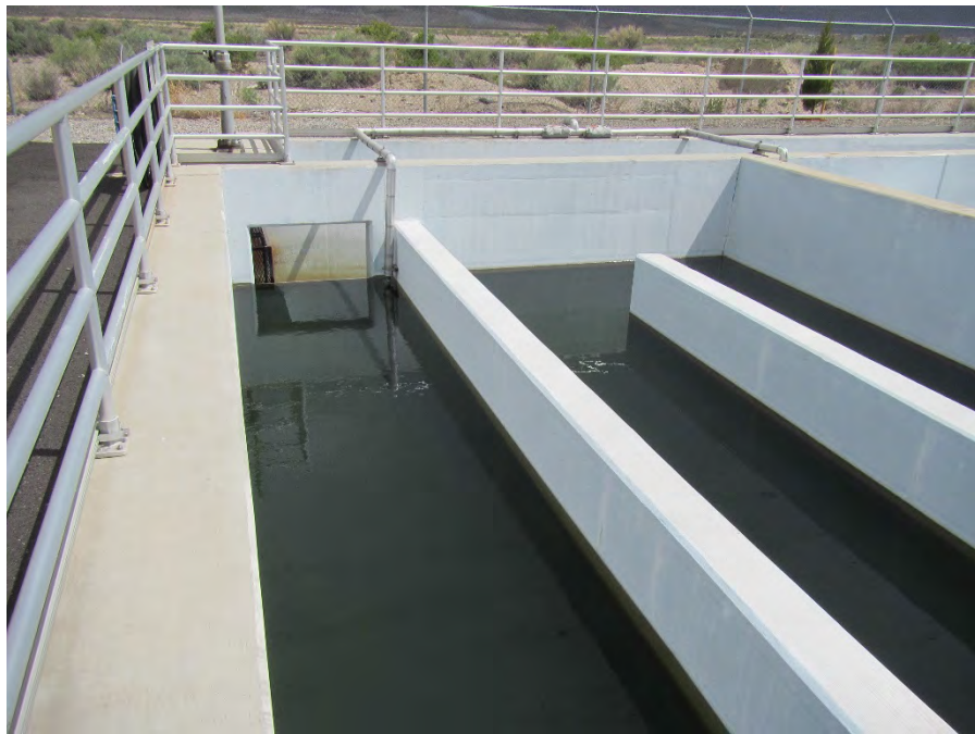
Photo 18 - Minor Concrete cracking at the Chlorine Contact Basin
