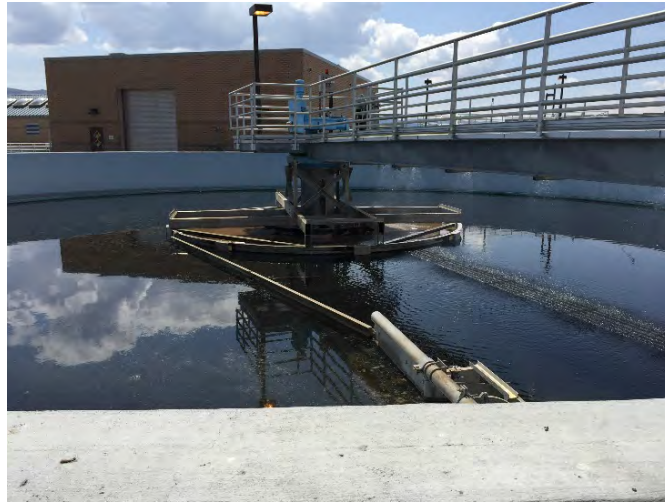
Photo 4.23 - Clarifier No. 3 Overall
