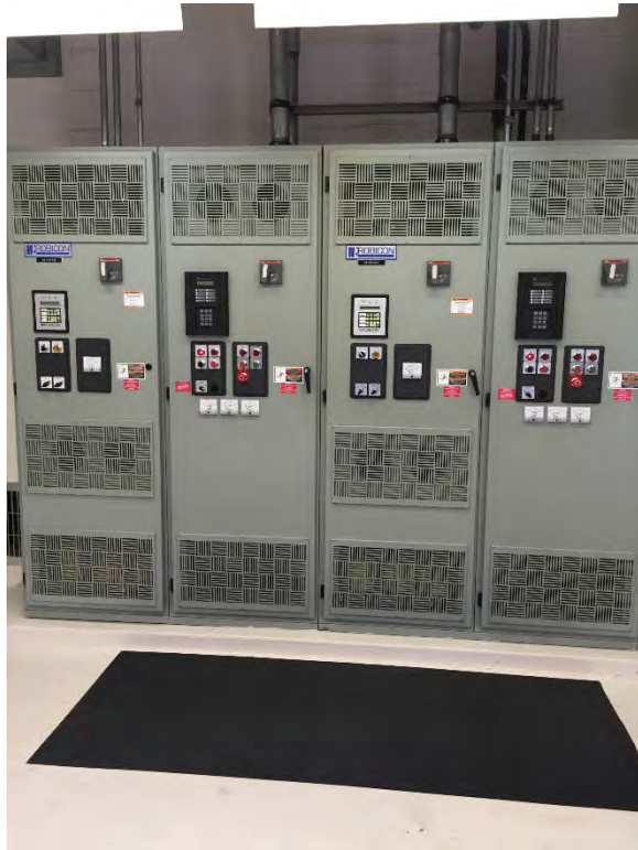
Photo 23 - Effluent Pump Station VFDs 4 and 5 are obsolete
