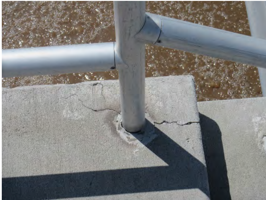
Photo 7 - Cracks at Oxidation Ditch
