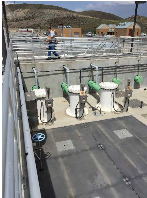
Photo 4.29 - Tertiary Filter Air Lift Pumps
