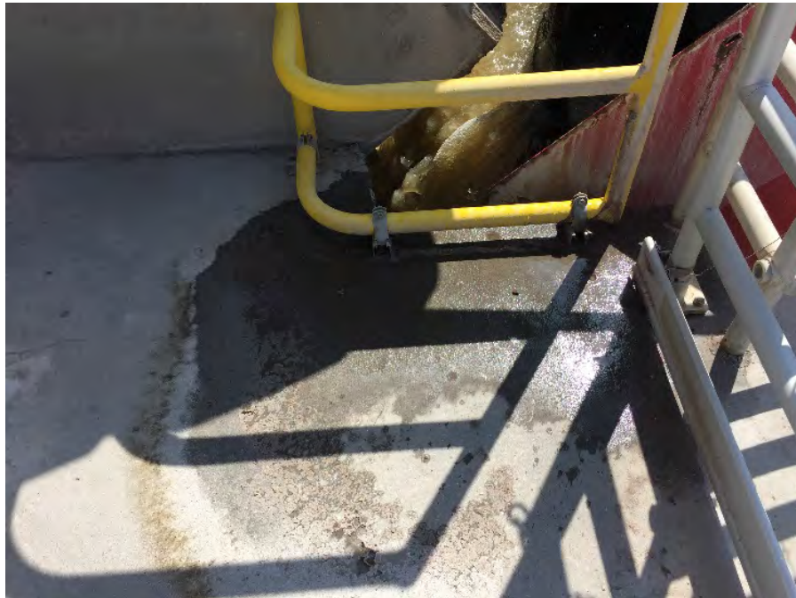
Photo 1 - Splashing occurs at the top of the lift pumps
