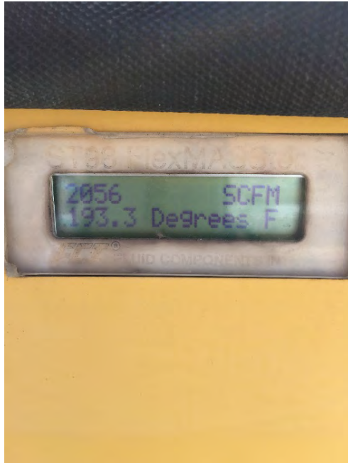
Photo 4.22 - Thermal Mass Air Flow Meter Readout
