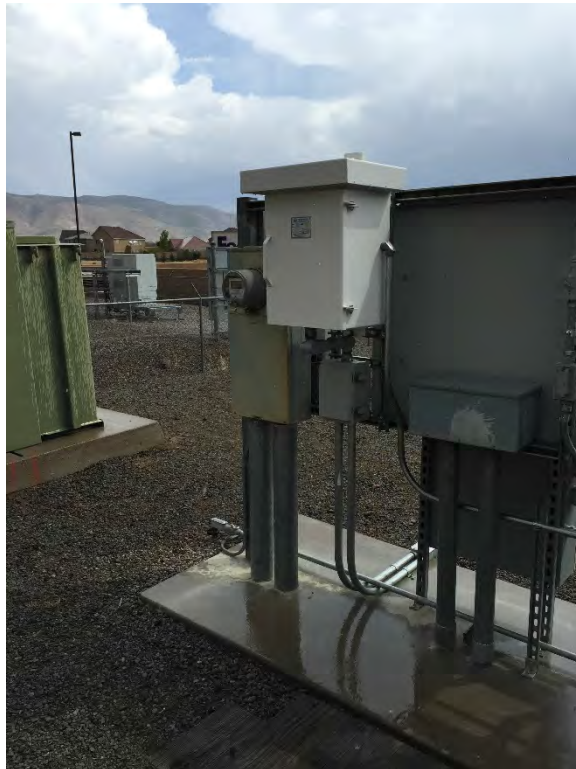
Photo 30 - Steamboat Creek Lift Station I & C equipment is obsolete
