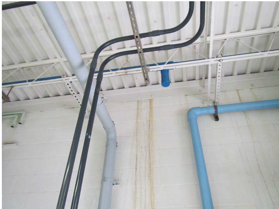
Photo 24 - Effluent Pump Station roof leak at the wall
