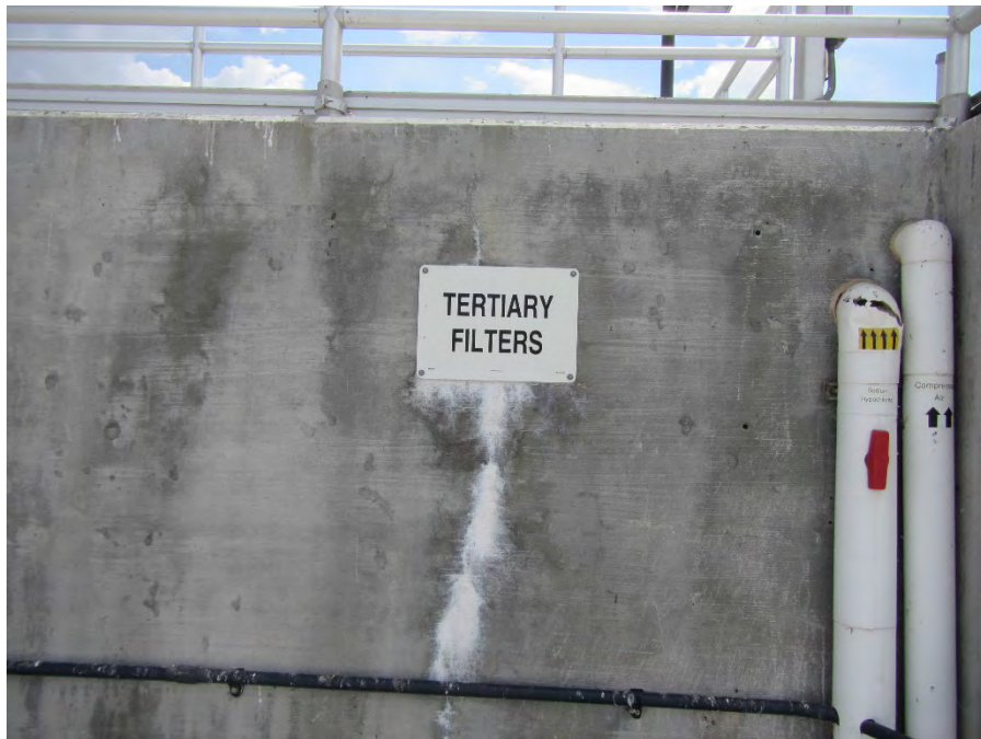
Photo 16 - Minor cracking of the concrete structure was observed at the Tertiary Filters
