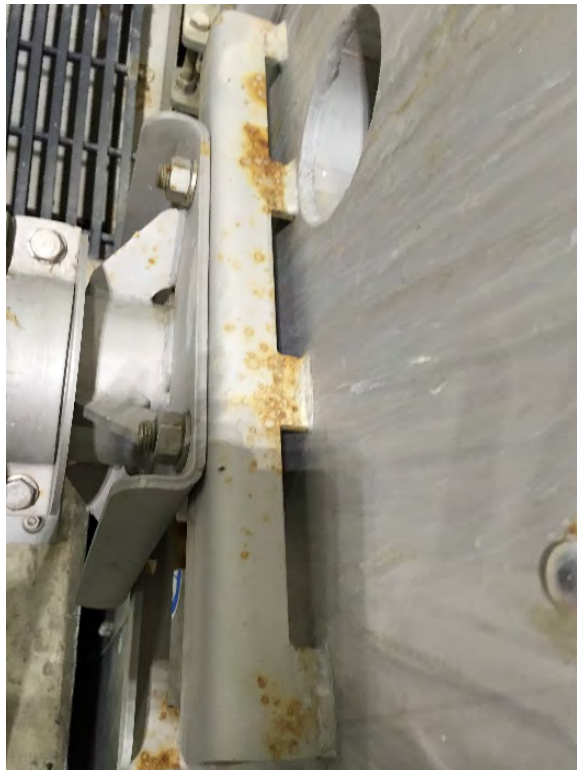
Photo 4 - Corrosion is accruing at various location on the screen and gates structure
