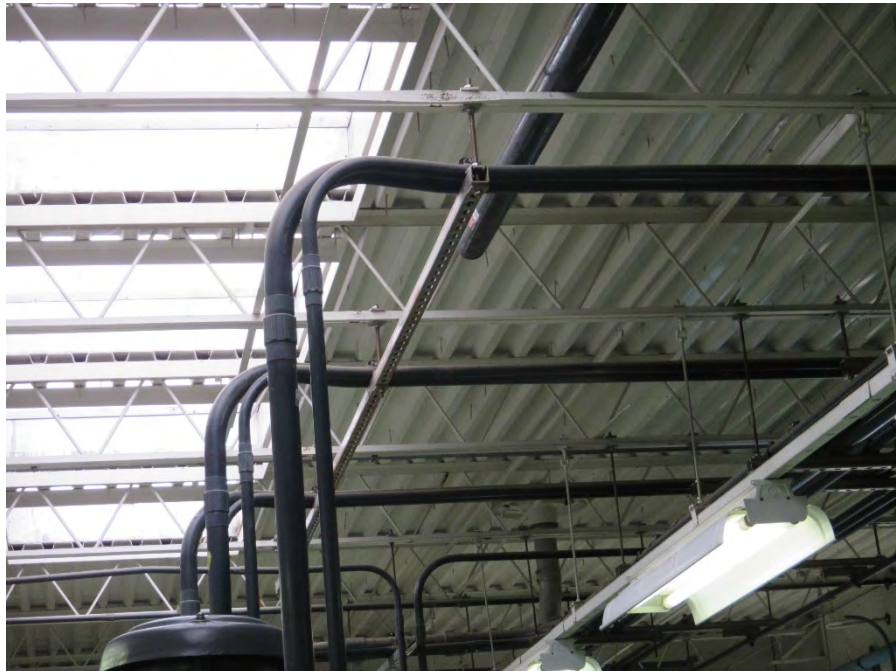
Photo 25 - Effluent Pump Station joist above Pump 1 is twisted at electrical conduit attachment
