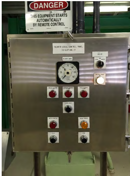
Photo 4.35 - Blower Local Control Panel
