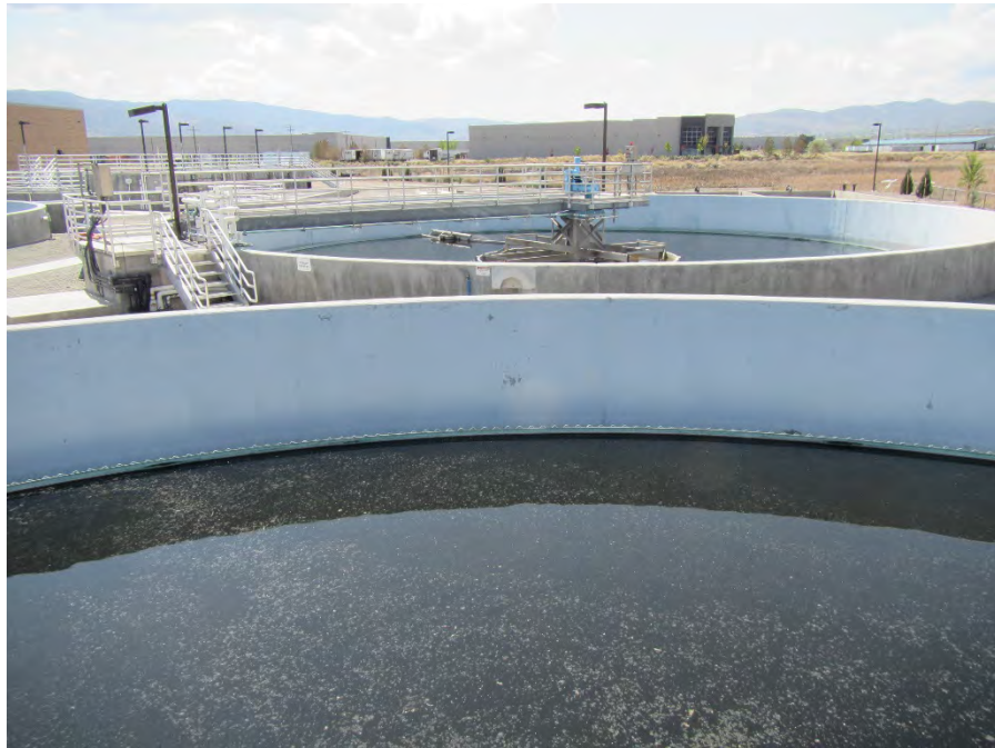
Photo 13 - Coating failure has occurred Secondary Clarifier No 2
