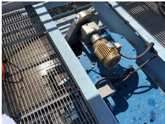
Photo 4.24 - Clarifier No. 1 Drive
