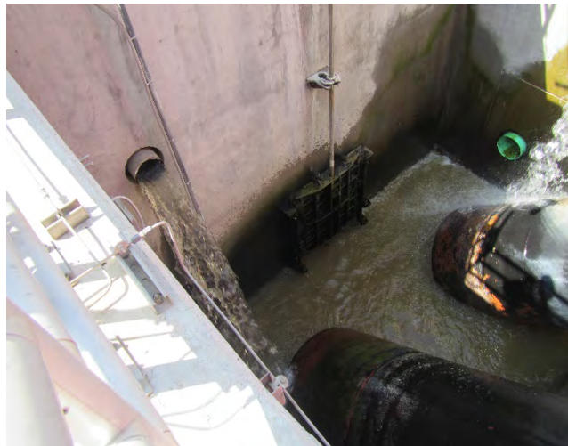
Photo 4.6 - Archimedes Screw Pump Suction Basin
