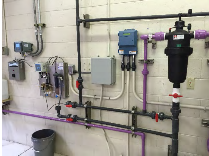
Photo 4.39 - Chlorine Contact Basins Chlorine Sampling Piping
