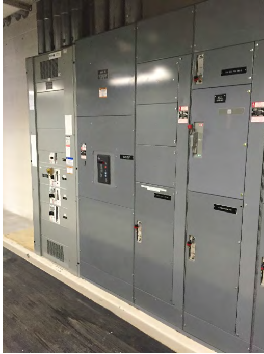
Photo 4.33 - Blower Electrical Room
