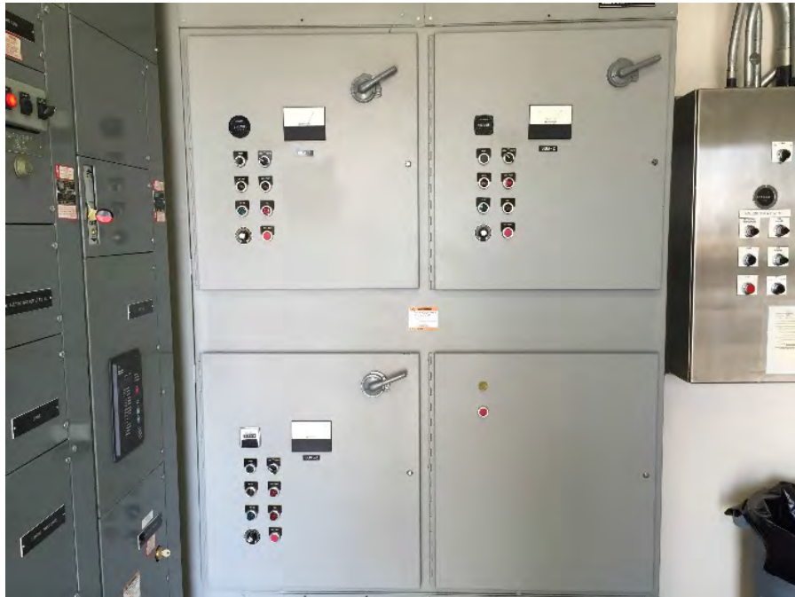
Photo 3 - VFDs Nos. 1, 2, 3, and 5 Mechanical mixers are obsolete
