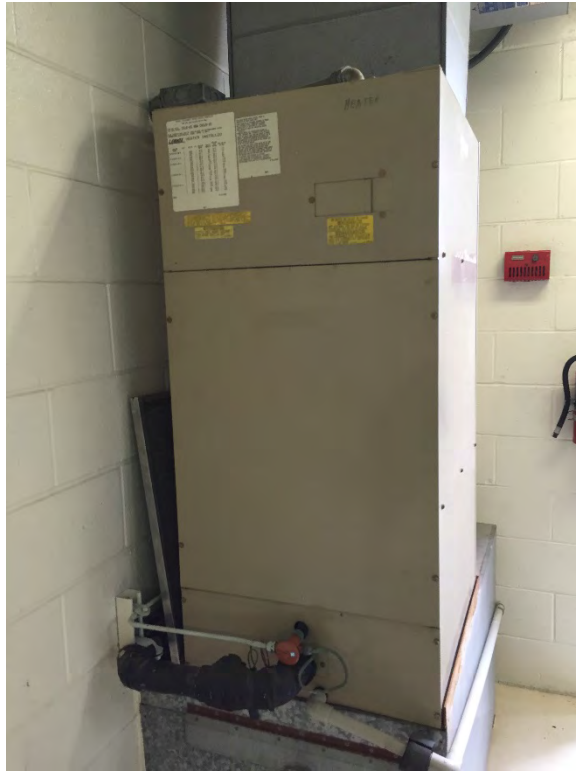
Photo 28 - Effluent Pump Station Electrical Room AC unit often freezes the evaporative coil within the air handler unit- Air Handler Unit
