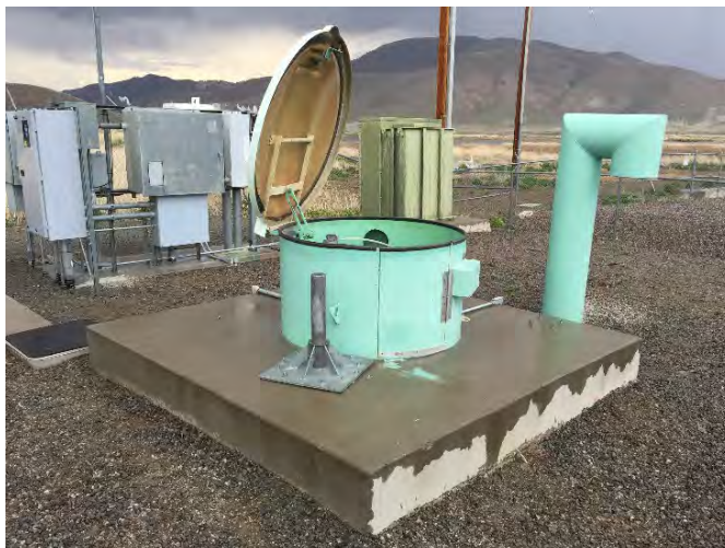
Photo 4.2 - SCLS Dry Well
