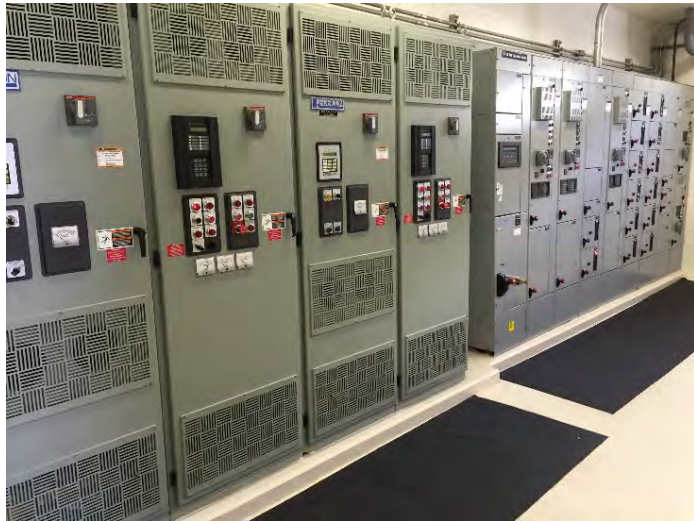
Photo 4.37 - RAS/WAS Electrical Room
