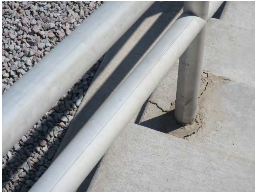
Photo 9 - Cracks at Oxidation Ditch
