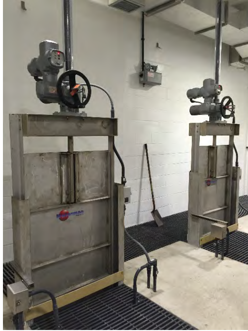
Photo 4.10 - Motor Operated Gates - Screens
