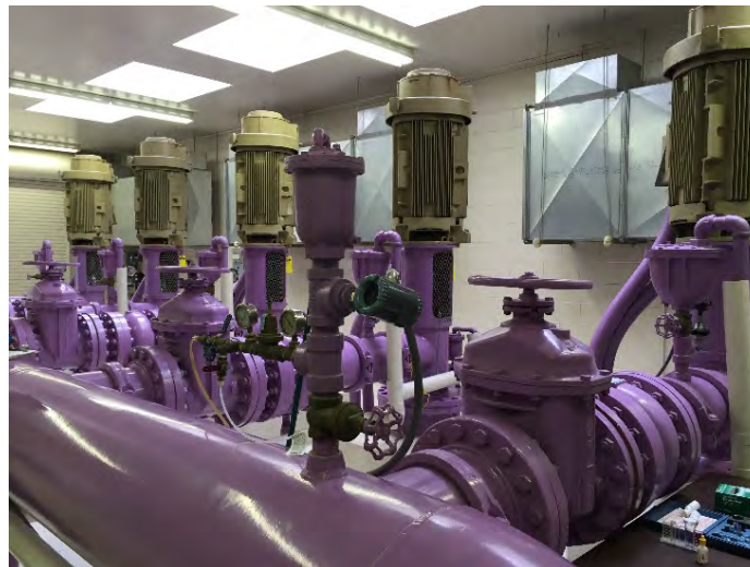
Photo 4.41 - Export Pump Station Vertical Turbine Pumps
