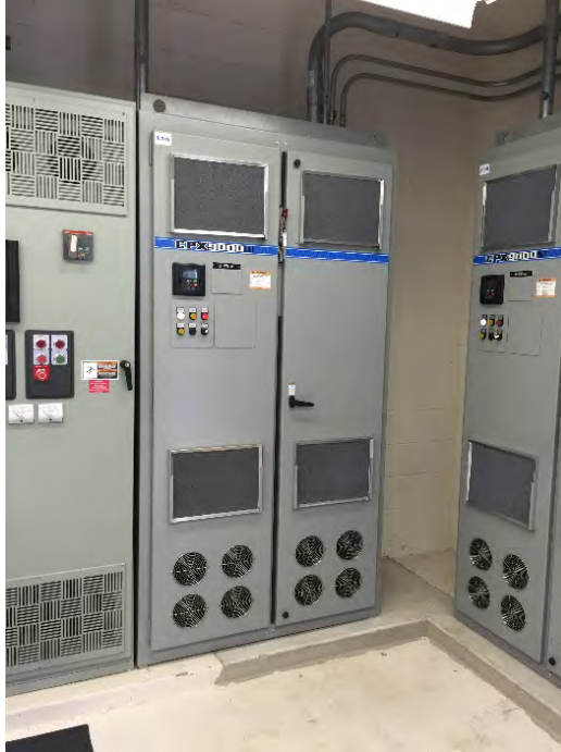
Photo 4.47 - Effluent Pump Station Variable Frequency Drive Nos. 1 and 2
