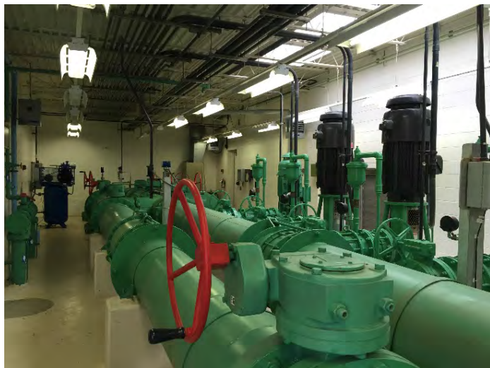
Photo 4.44 - Effluent Pump Station Vertical Turbine Pumps
