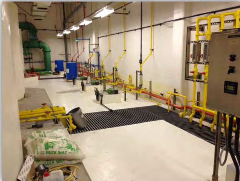
Photo 4 Sodium Hypochlorite and Alum Piping North Interior Wall of CSB
