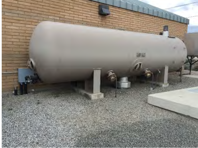
Photo 4.42 - Export Pump Station Surge Tank
