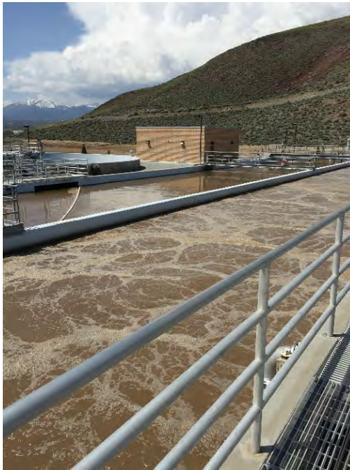
Photo 4.17 - Fine Bubble Aeration
