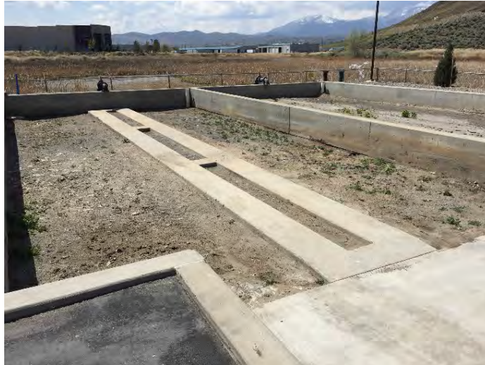
Photo 4.50 - Sand Drying Beds
