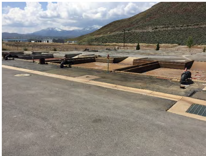
Photo 4.51 - Sludge Dewatering Beds
