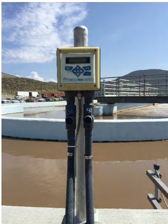
Photo 11 - Some of the local meter panels do not have sun shade protection at the Oxidation Ditch
