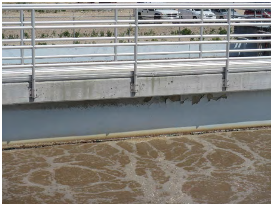
Photo 6 - Coating failure has occurred at the Oxidation Ditch
