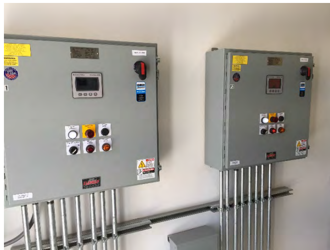
Photo 4.9 - Mechanical Screen Control Panels
