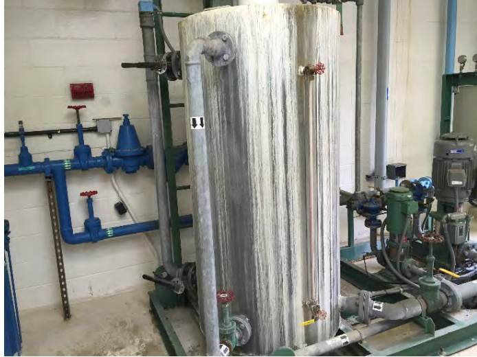
Photo 4.49 - Plant Water Booster Station
