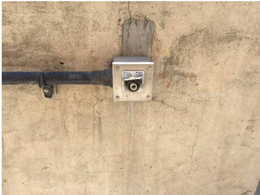
Photo 2 - IPS Damage Emergency Stop Button
