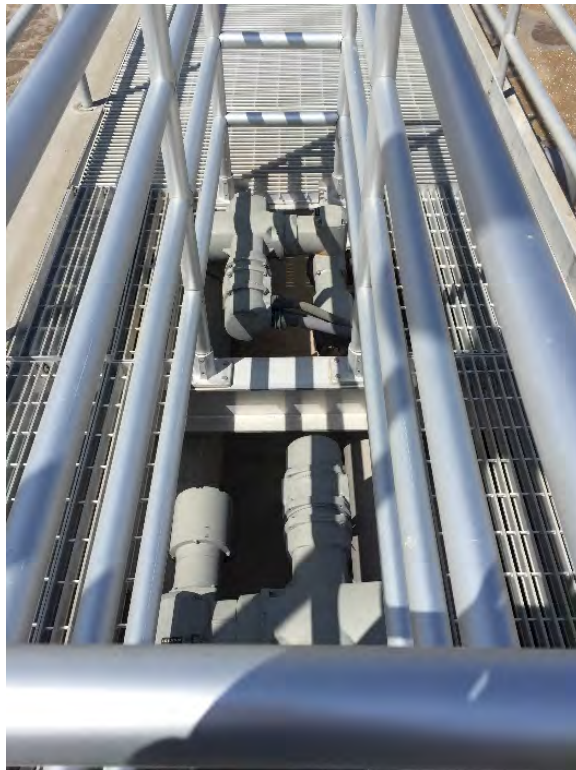
Photo 10 - Air Leaks at Aeration Piping
