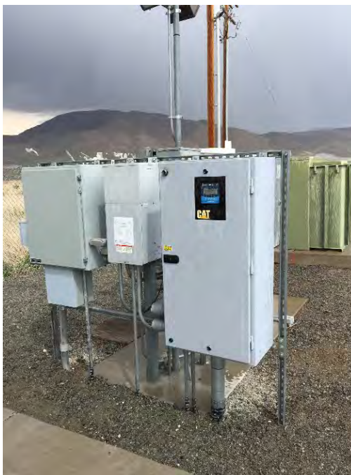
Photo 4.3 - SCLS Local Control Panel
