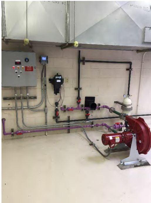
Photo 4.40 - Chlorine Contact Basins Turbidity Sample Pump and Piping
