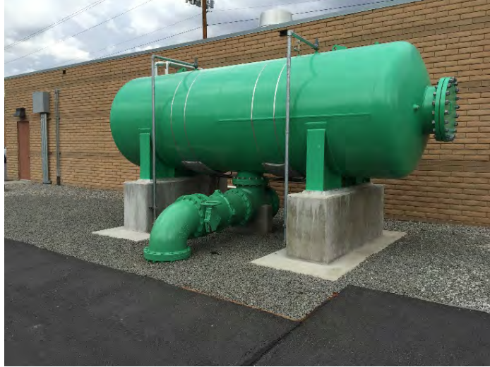
Photo 4.45 - Effluent Pump Station Surge Tank
