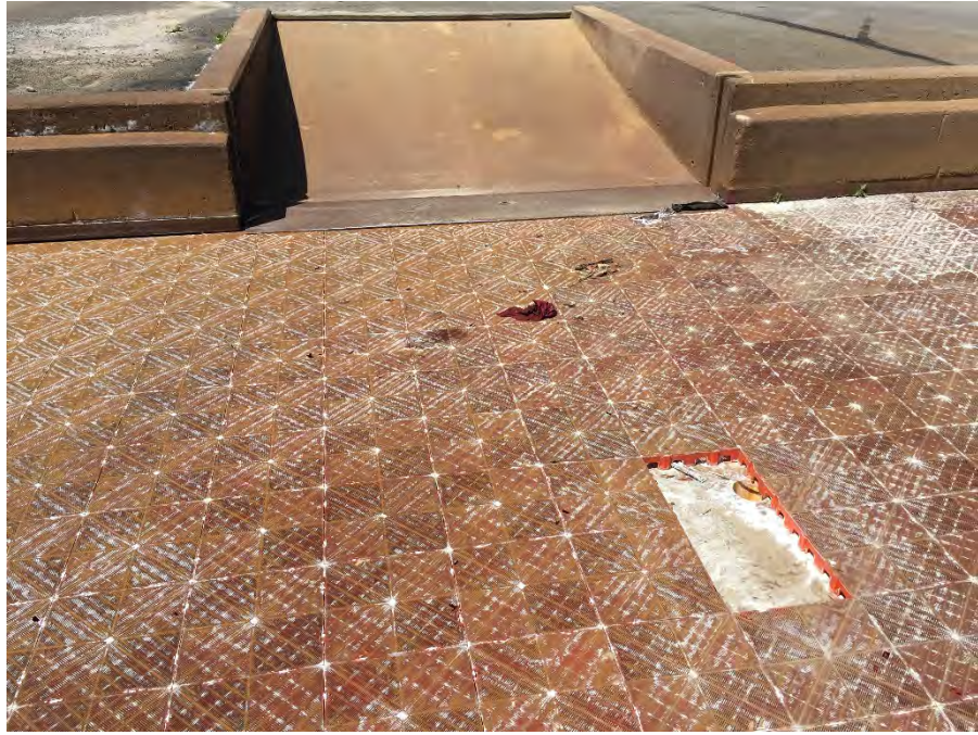
Photo 29 - The Sand Drying and Sludge Dewatering Beds are degraded
