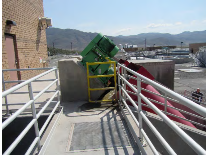
Photo 4.7 - Archimedes Screw Pump Drives
