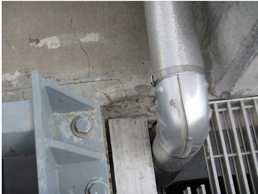
Photo 17 - Minor Concrete cracking at the Chlorine Contact Basin
