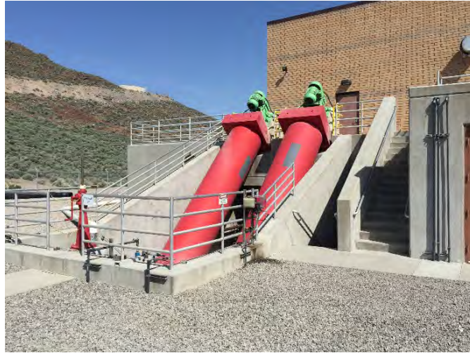
Photo 4.5 - Overall View Influent Pumping Station
