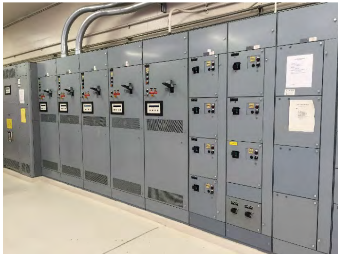
Photo 4.43 - Export Pump Station Electrical Equipment
