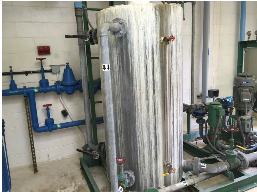
Photo 22 - NPW Station should cleaned and preserved
