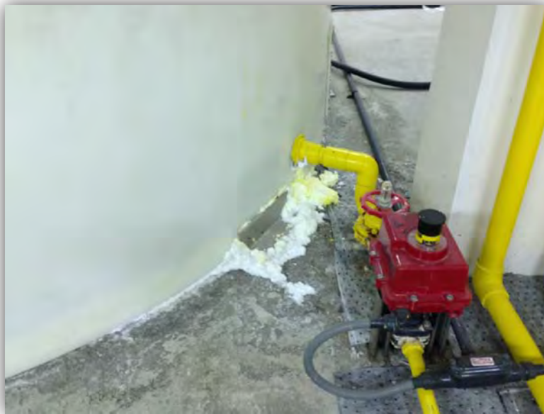
Photo 5 Sodium Hypochlorite Piping and Fittings at the Suction of the Sodium Hypochlorite Tank
