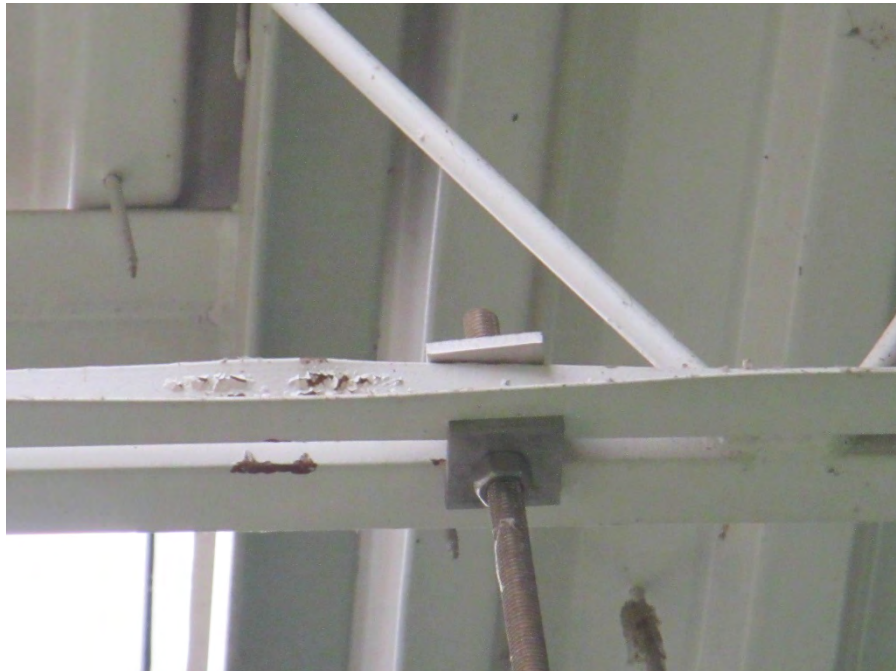
Photo 26 - Effluent Pump Station joist above Pump 1 is twisted at electrical conduit attachment
