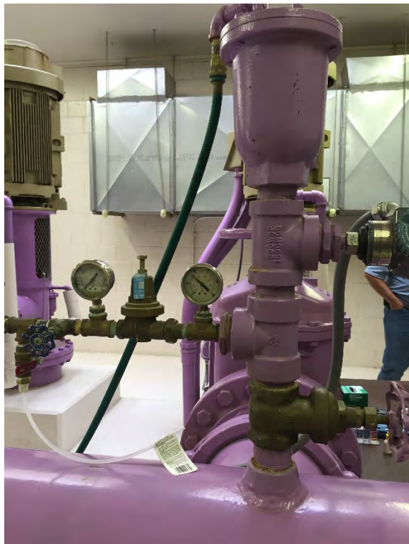
Photo 21 - Air release valves have garden hose vice hard piping to the floor drains
